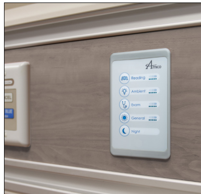
Lights Controlled at Headwall
