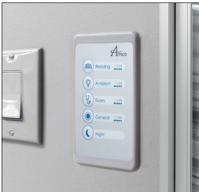
Lights Controlled at Patient Room Door
