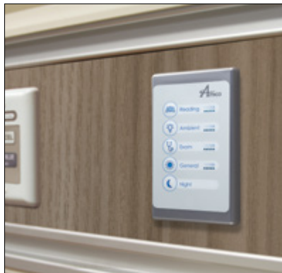
Lights Controlled at Headwall
