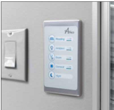
Lights Controlled at Patient Room Door
